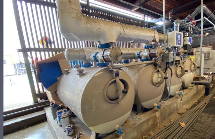
West Campus Pool Filter
