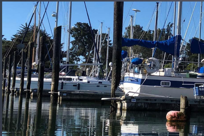
Decaying Timber Piles
