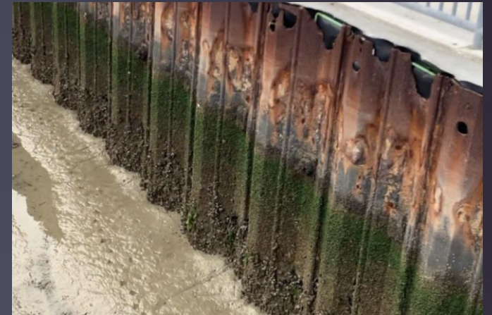
Aged Sheet Pile Wall - South Cove
